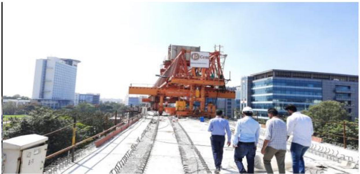
Industrial Visit: Students from M.tech Structures & Transportation, Civil Engineering Department, MVJCE, Hoodi R-1 reach at BMRCL
