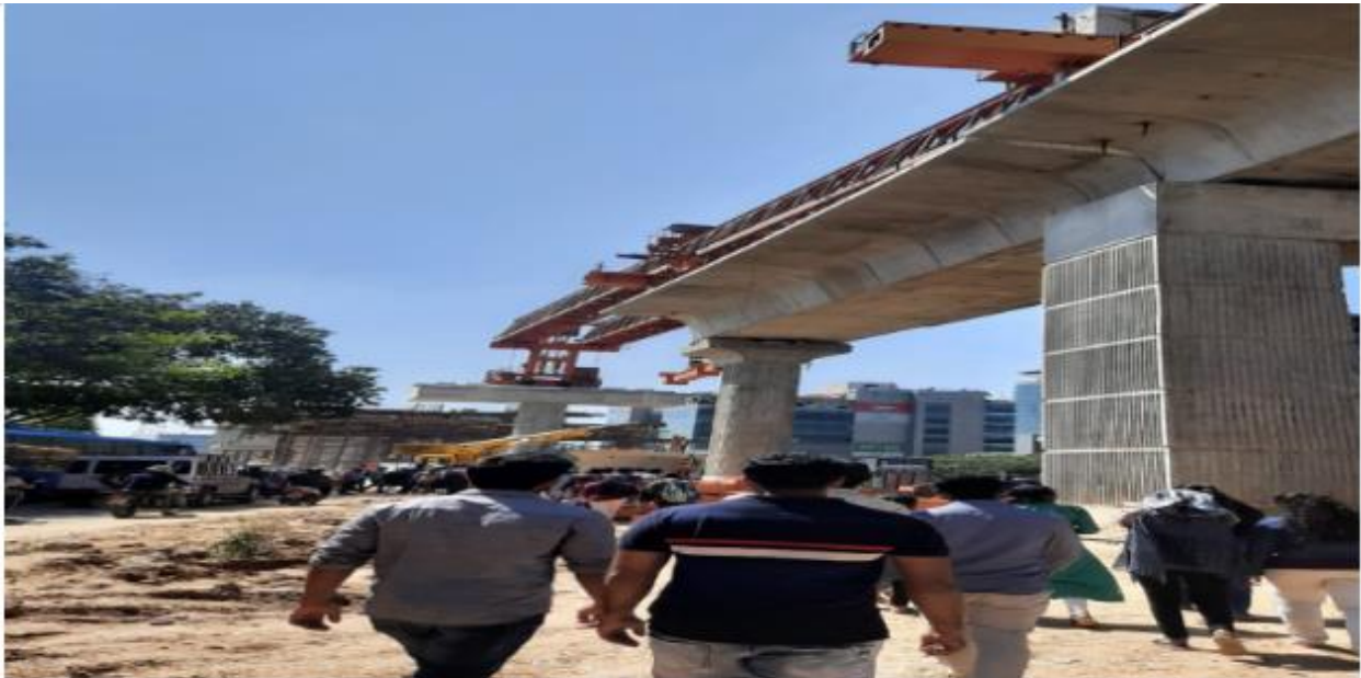
Industrial Visit: Students from M.tech Structures & Transportation, Civil Engineering Department, MVJCE, Hoodi R-1 reach at BMRCL visiting erection of precast elements on 04/11/2019
