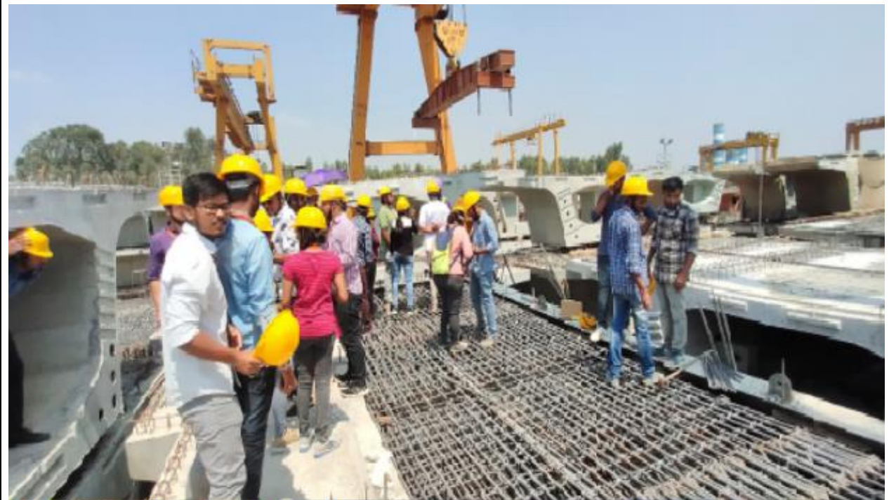
Industrial Visit:Mr.Shishir Kumar, site manager,briefing about the details of Reinforcements to Civil Engineering students,MVJCE at BMRCL(Whitefield-Baiyappanahalli Reach-1) Bengaluru on 11/04/2019
